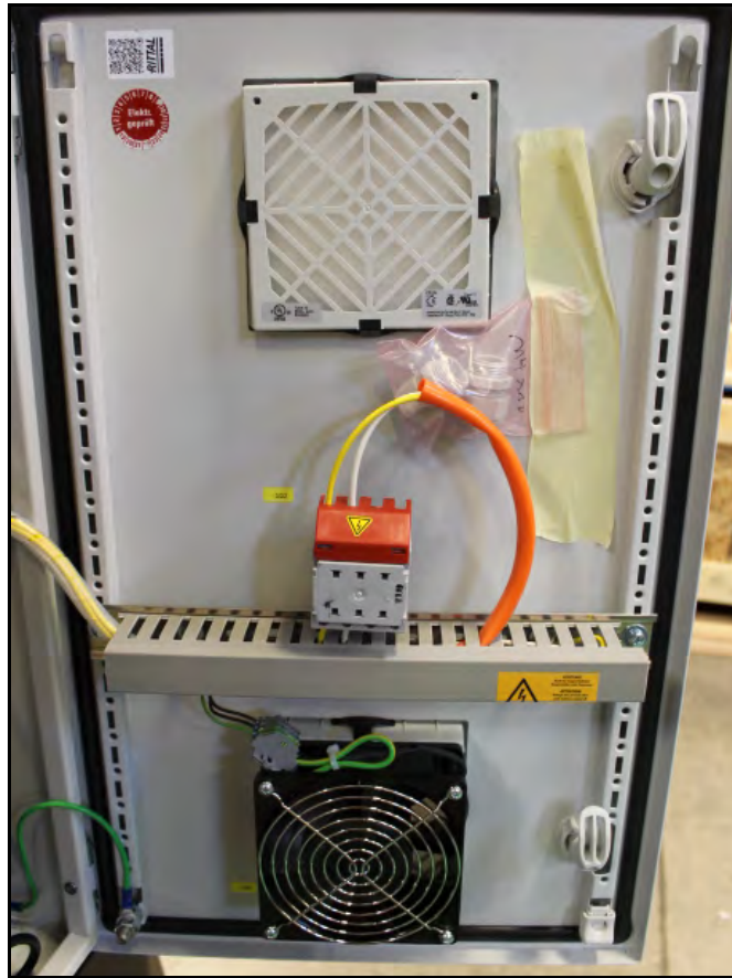
Figure 34 Control Box Filter (inside)
