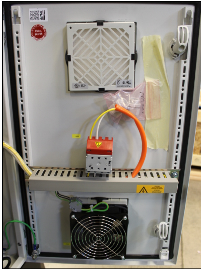
Figure 34 Control Box Filter (inside)
