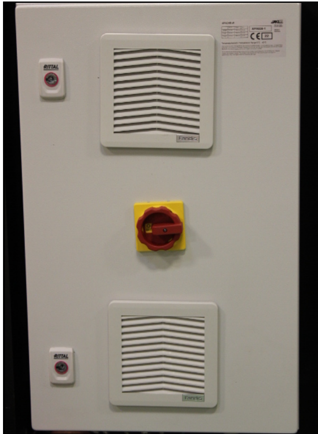
Figure 33 Control Box Filter
