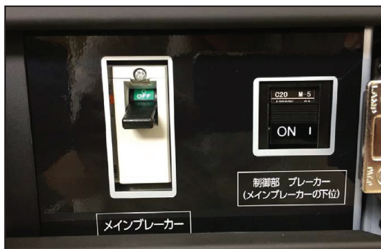
Figure 177 Control box - Main breaker
