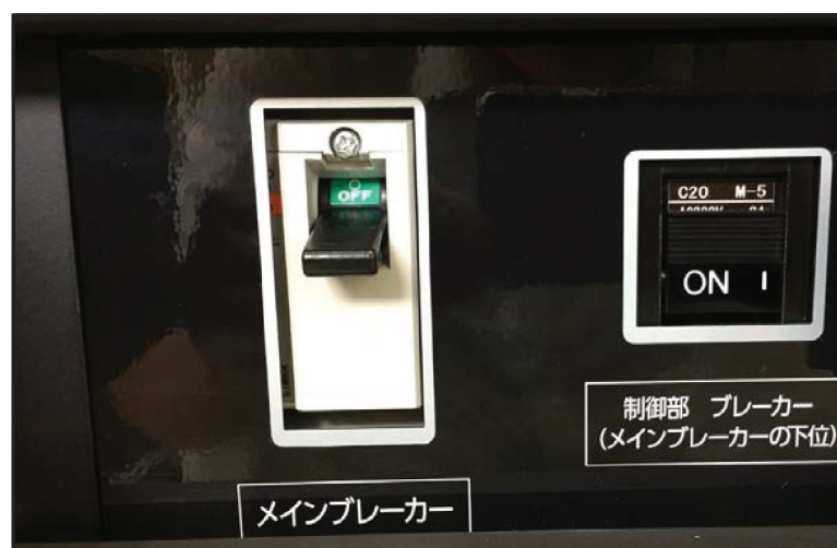
Figure 188 A/D BOX - Main breaker
