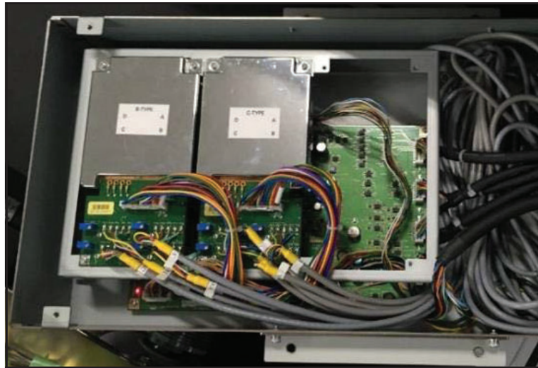
Figure 200 A/D BOX - A/D box cover removed
