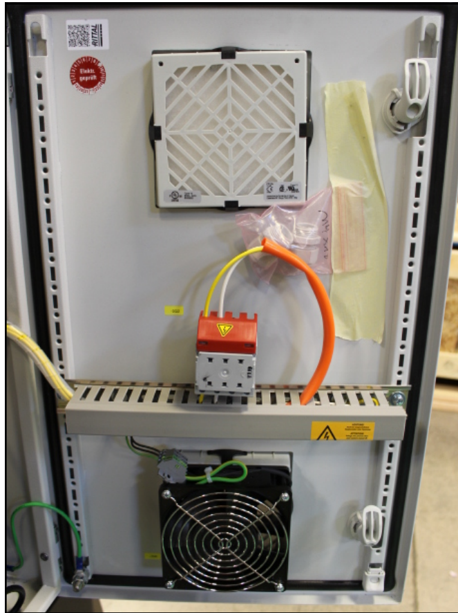
Figure 22 Control Box Filter (inside)
